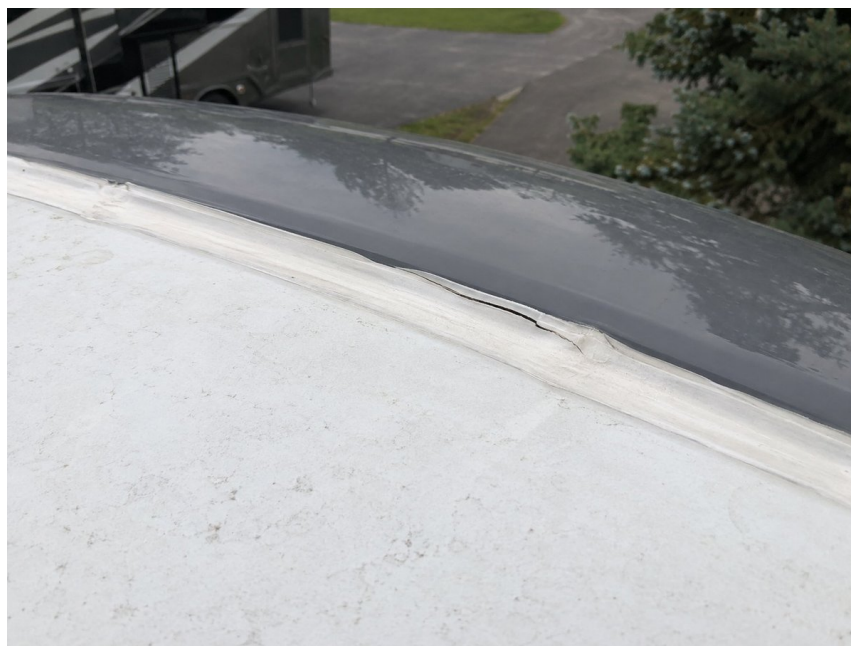
Illustration: Separation along the front cap-to-roof sealant joint.
