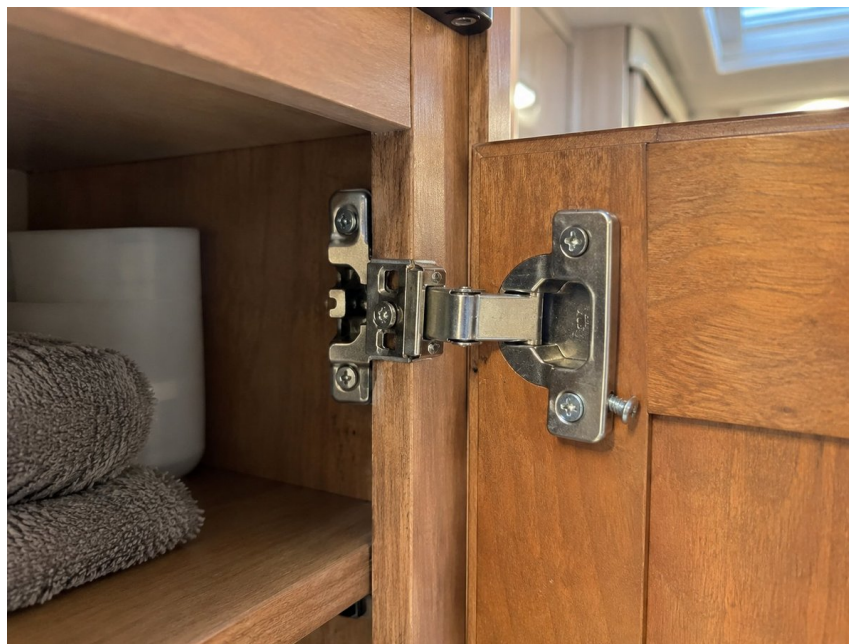
Illustration: Loose bathroom cabinet hinge mounting.
