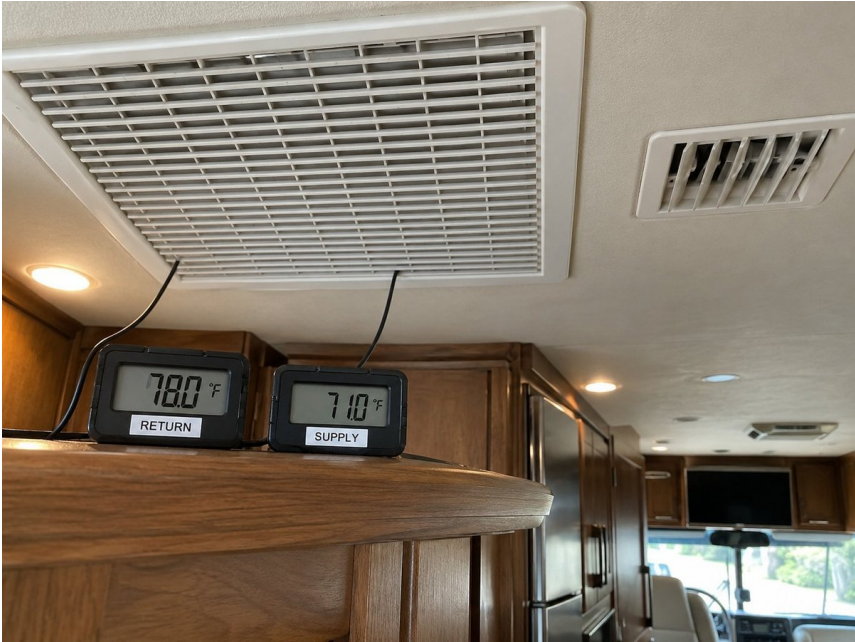
Illustration: Interior return and supply temperature test setup: 78 F and 71 F.
