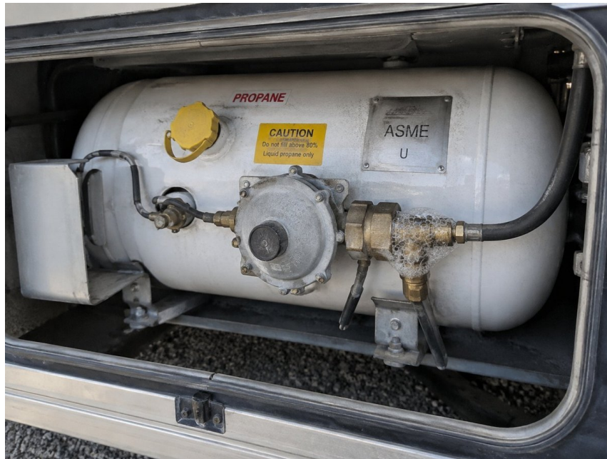
Illustration: ASME tank and accessible regulator outlet connection.
