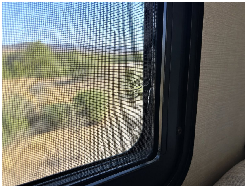
Illustration: Tear in the bedroom window screen mesh.
