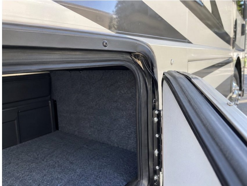
Illustration: Separated storage-door weather seal at the upper corner.
