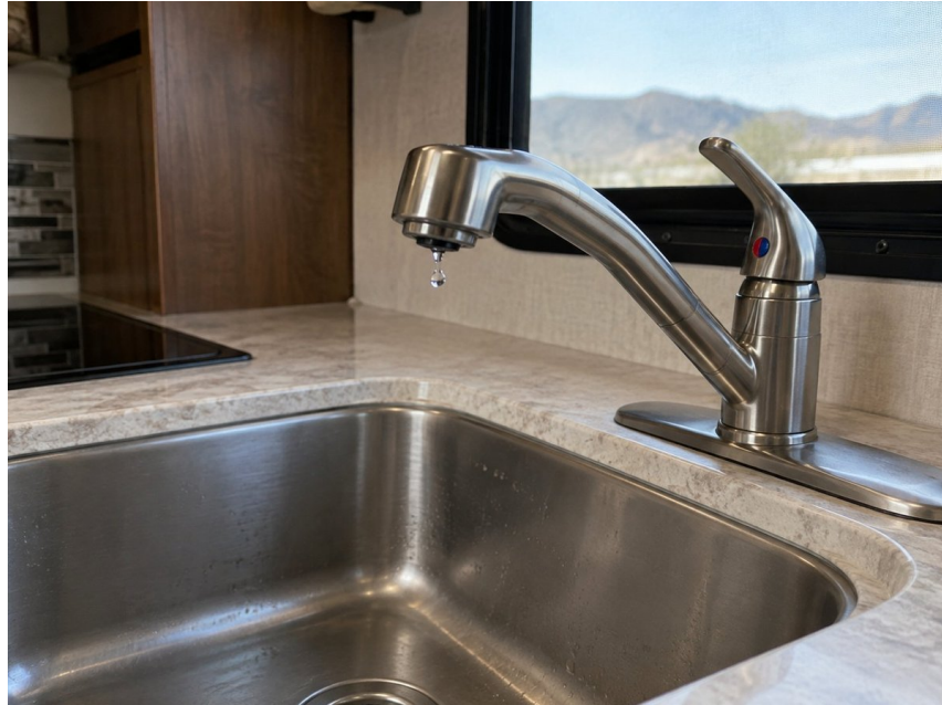
Illustration: Drip at the kitchen faucet spout after shutoff.
