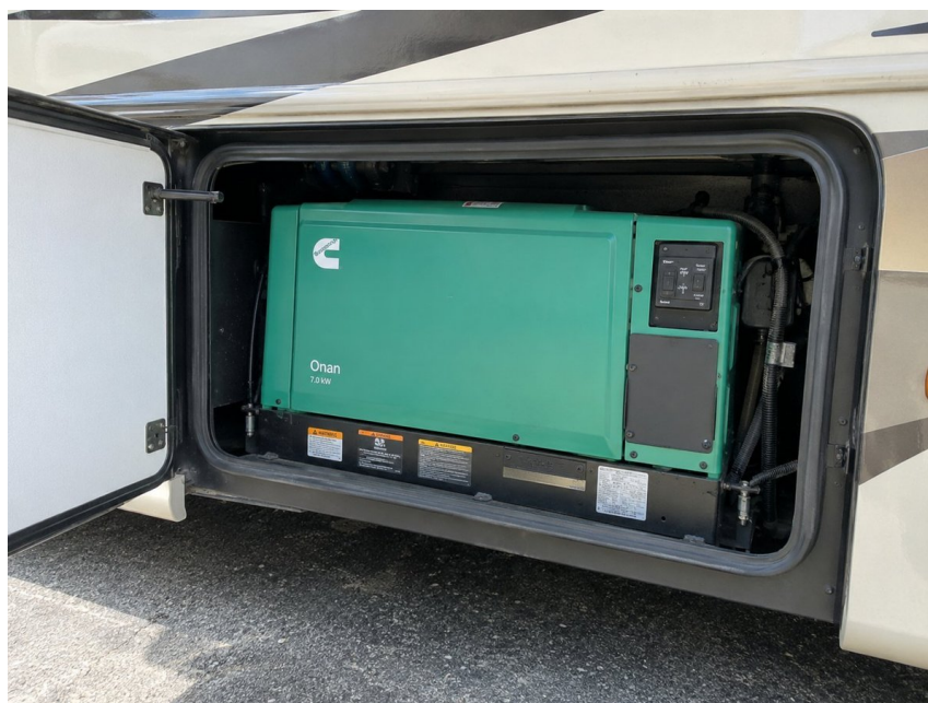
Illustration: Gasoline generator compartment; the loaded shutdown is described above.
