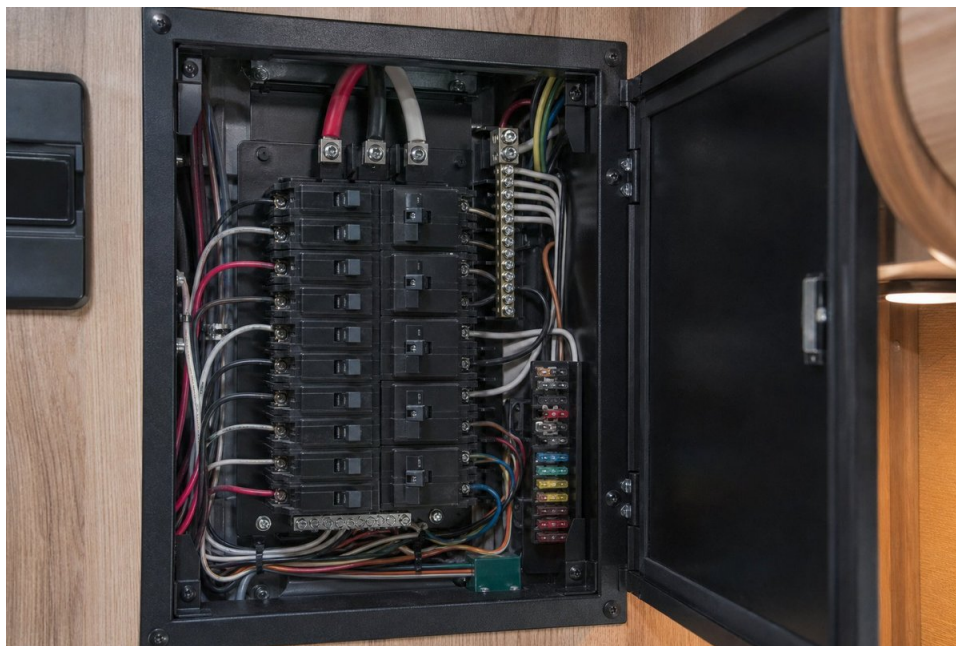
Illustration: Accessible electrical distribution panel overview
