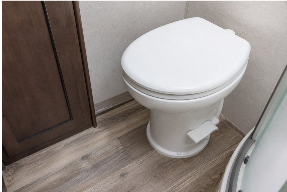
Illustration: Toilet and visible water connection
